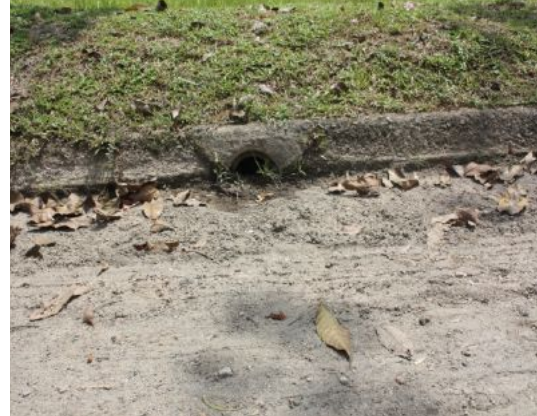
Gambar 1.42 Scupper Drain Dipenuhi Pasir
